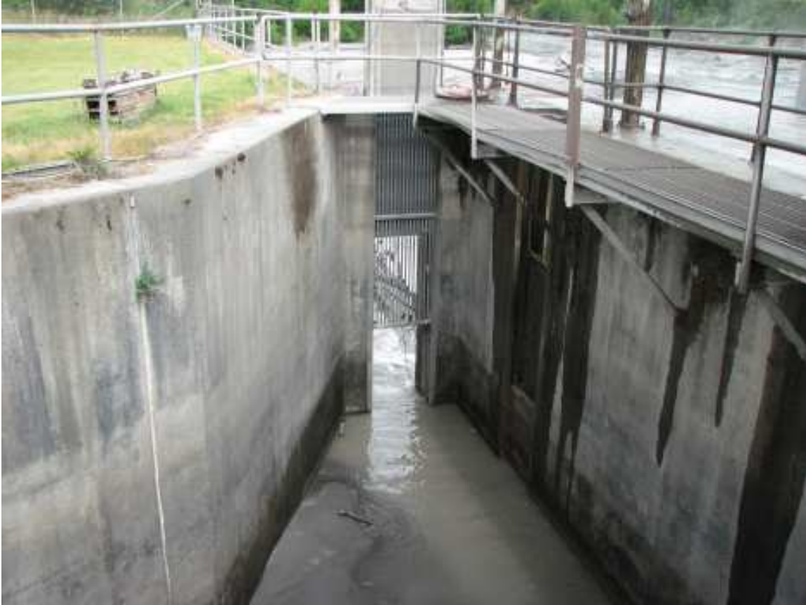
Figure 20 Two of the three gates: the existing single-functional gate and the currently blocked off gate to its right.
