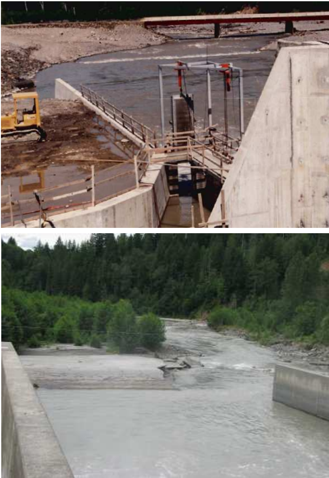
Figure 25 Photographs of original construction (5/89) (top) (Source: USACE) and current conditions (6/09) show the tailwater feature from the upstream side.
