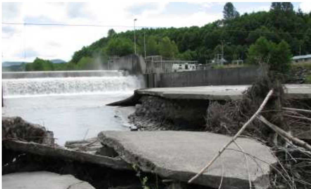
Figure 26 Photographs of the original construction (6/89) (top) (source: USACE) and of current conditions (6/09) show the tailwater feature from the downstream side. These pictures show very graphically the downstream sill degradation and breach of the right end and the lower resulting tailwater.
