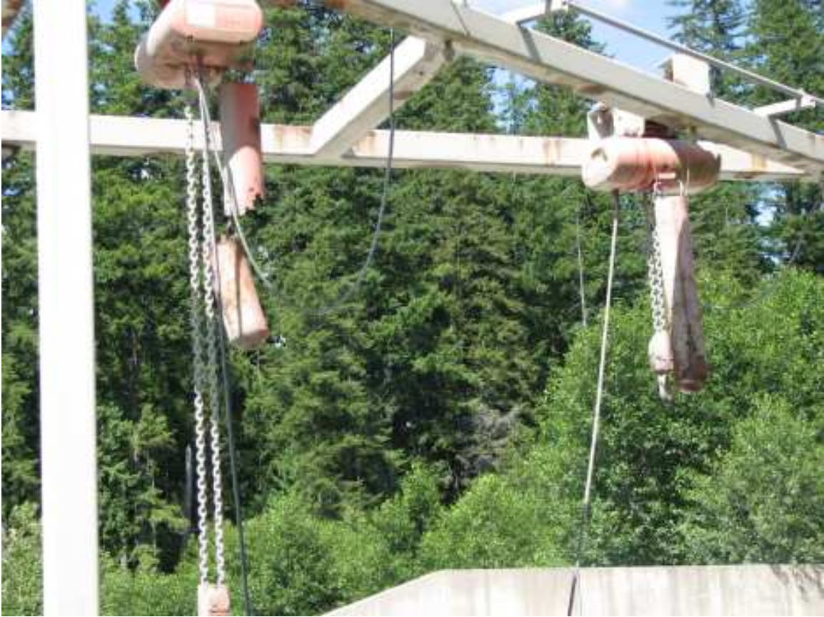
Figure 21 Marginally functional gate lifts and chain cans.
