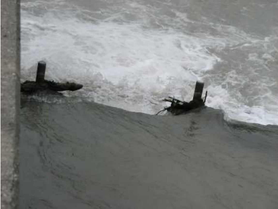
Figure 19 Existing stoplog bay obstructed by debris accumulating on opening and stoplog supports.
