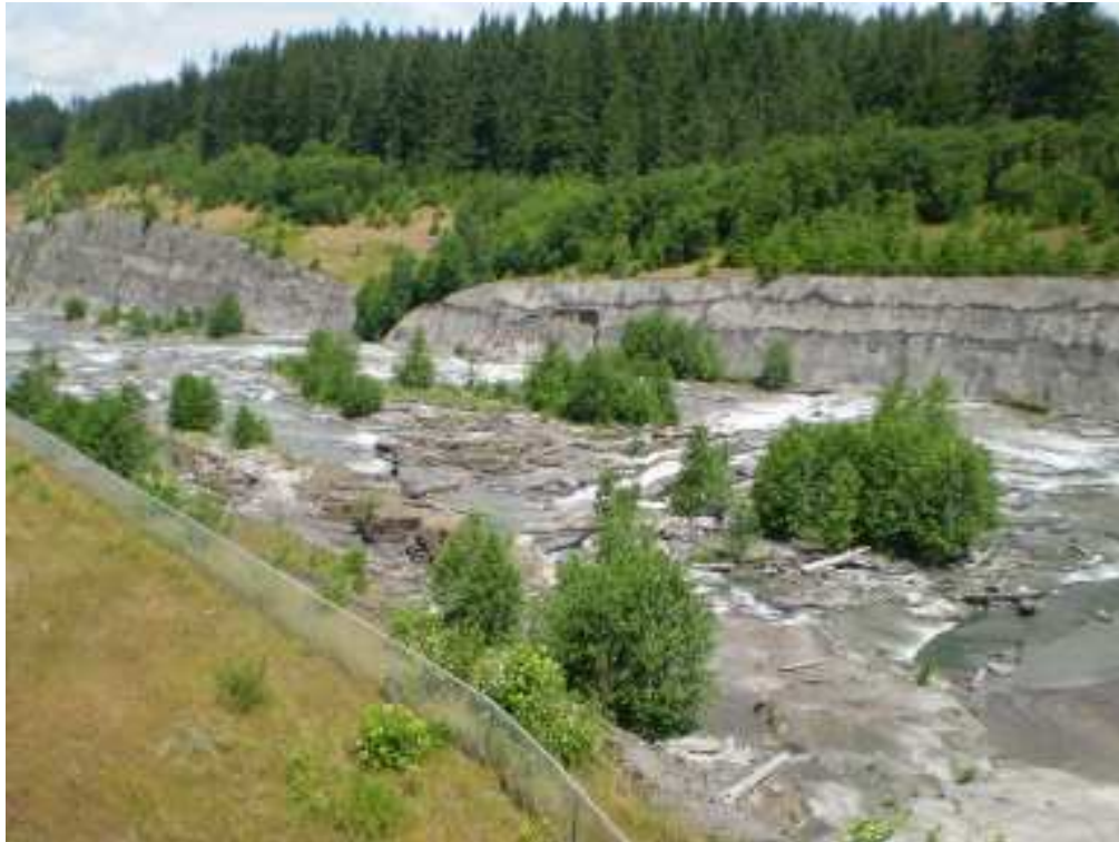
Figure 30 Spillway (note fractured concrete apron) and rock ramp at SRS.
