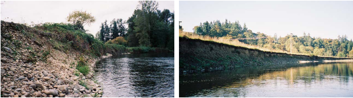
Figure 4. 32. Rapidly eroding terraces at RM 10.9 (left) and RM 9.5 (right). These rapidly eroding banks present good restoration opportunities.
