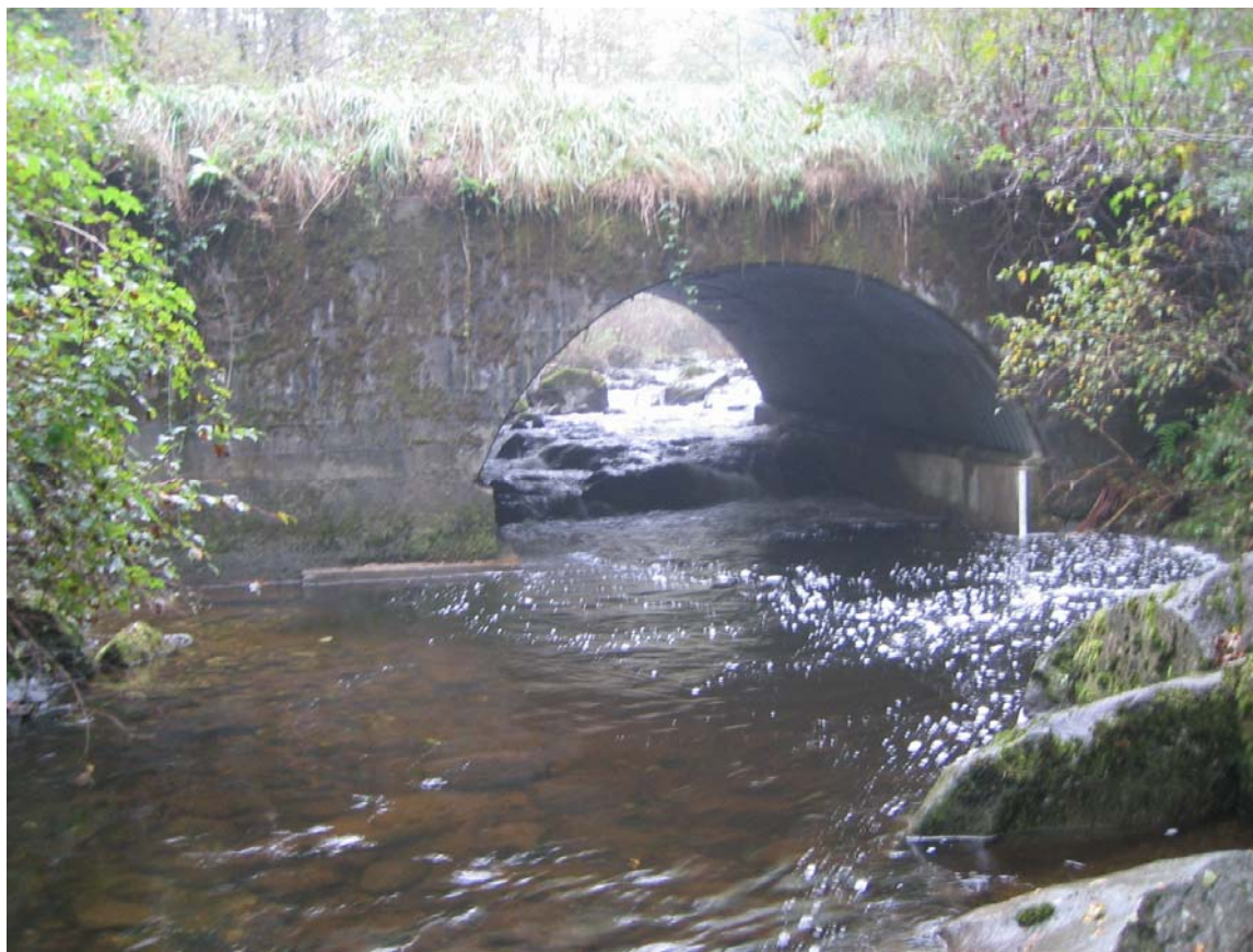
Figure 4. 120. Picture of culvert beneath USFS Road 42, 66m upstream from the mouth of Slide Creek.
