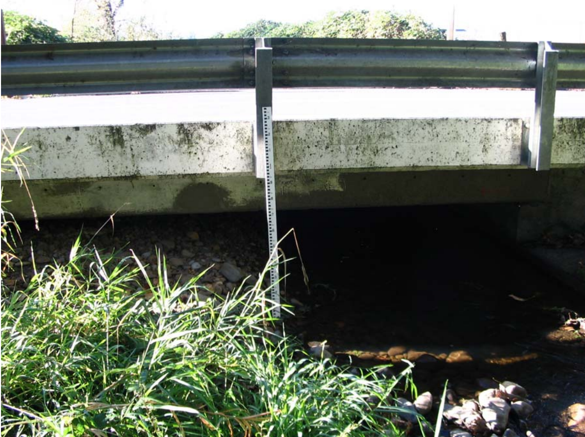
Figure 4. 84. Picture of bridge over Dean Creek at the upstream end of the survey area.
