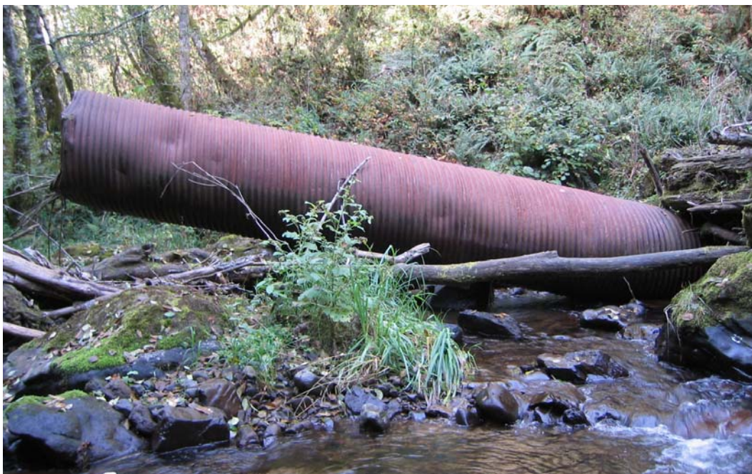
Figure 4. 111. Photo of washed out culvert in the stream channel approximately 1000m from the mouth of King Creek.
