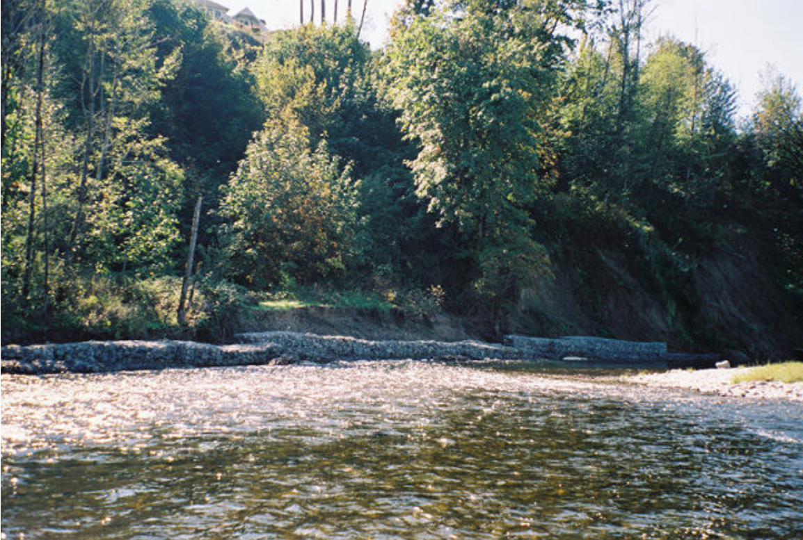
Figure 4. 5. Rock filled wire basket gabions protecting toe of eroding streambank at river mile 8.7 on the East Fork Lewis River. Photo taken September 2004
