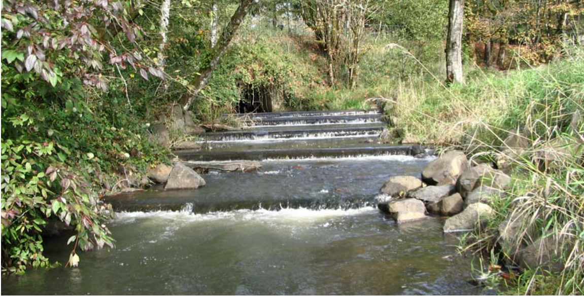
Figure 4. 74. Set of weirs set up to improve passage through the County Road 42 culvert. Note rip rap on both banks.
