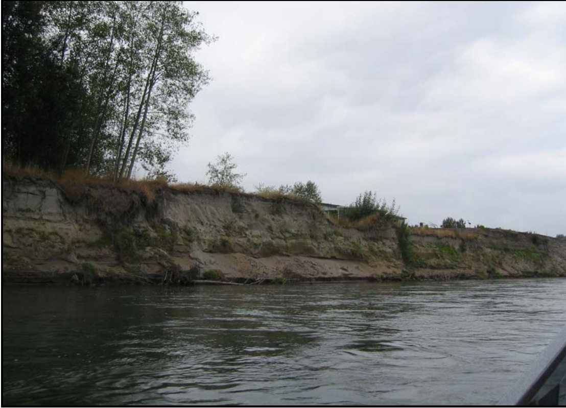
Image looking towards left bank at Horseshoe Bend near RM 13.5. (Photo from 2006, much of this bank has been armored with riprap in 2007)
