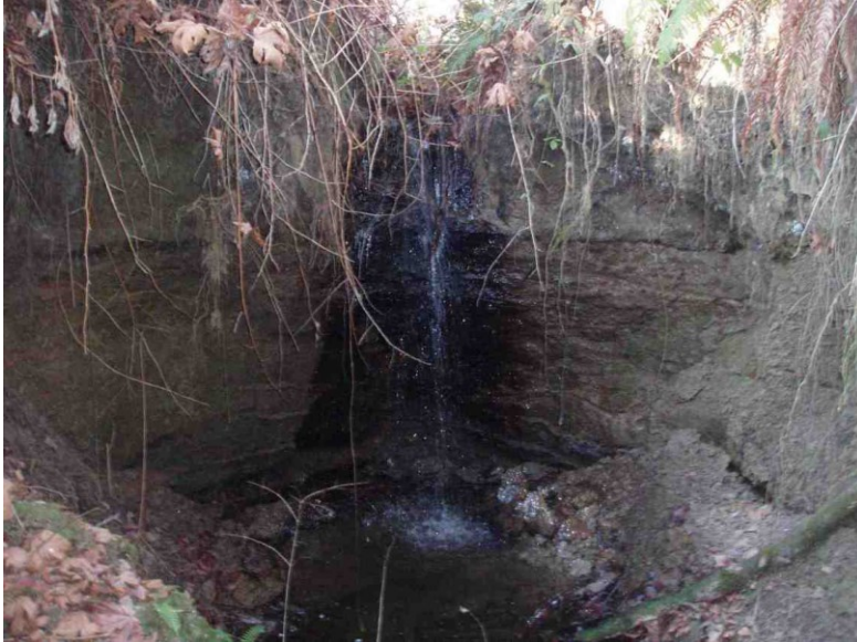
Figure 25. Photo of headcut just downstream of outlet of stormwater detention facility at headwaters of Trib W8.36. Approximate height of headcut is 6 feet.
