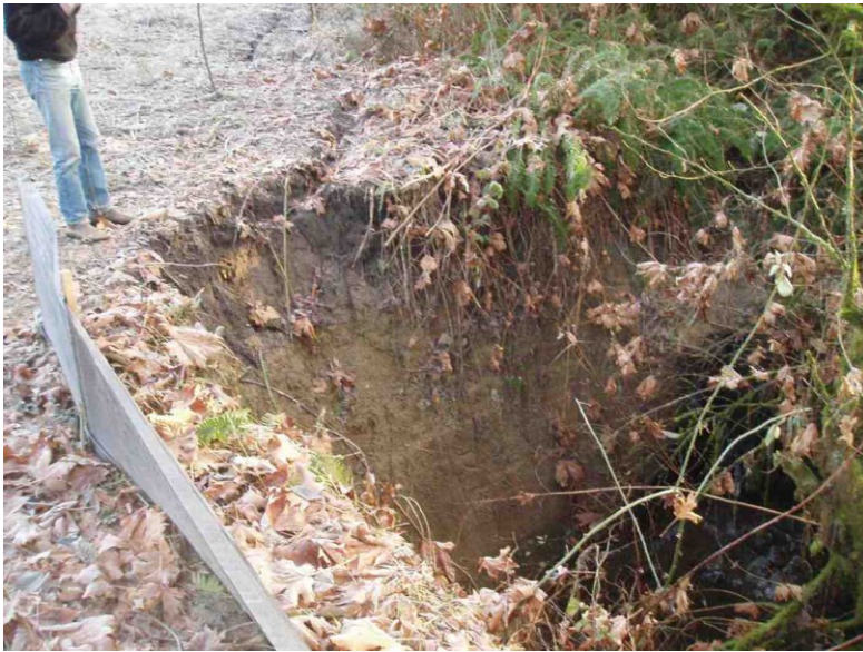
Figure 24. Photo of headcut just downstream of outlet of stormwater detention facility at headwaters of Trib W6.44 (Clark County Fairgrounds site). Approximate height of headcut is 12 feet.
