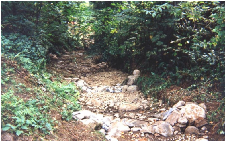
Figure 47. Series of rock grade control/headcut revetment structures placed in Oak Creek, Portland, OR
