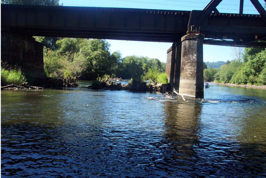
Photo 9 – View downstream under RR Bridge. There is a lot of LWD submerged on the left bank and along the left bank of the channel downstream. Fishing access is along the right bank.
