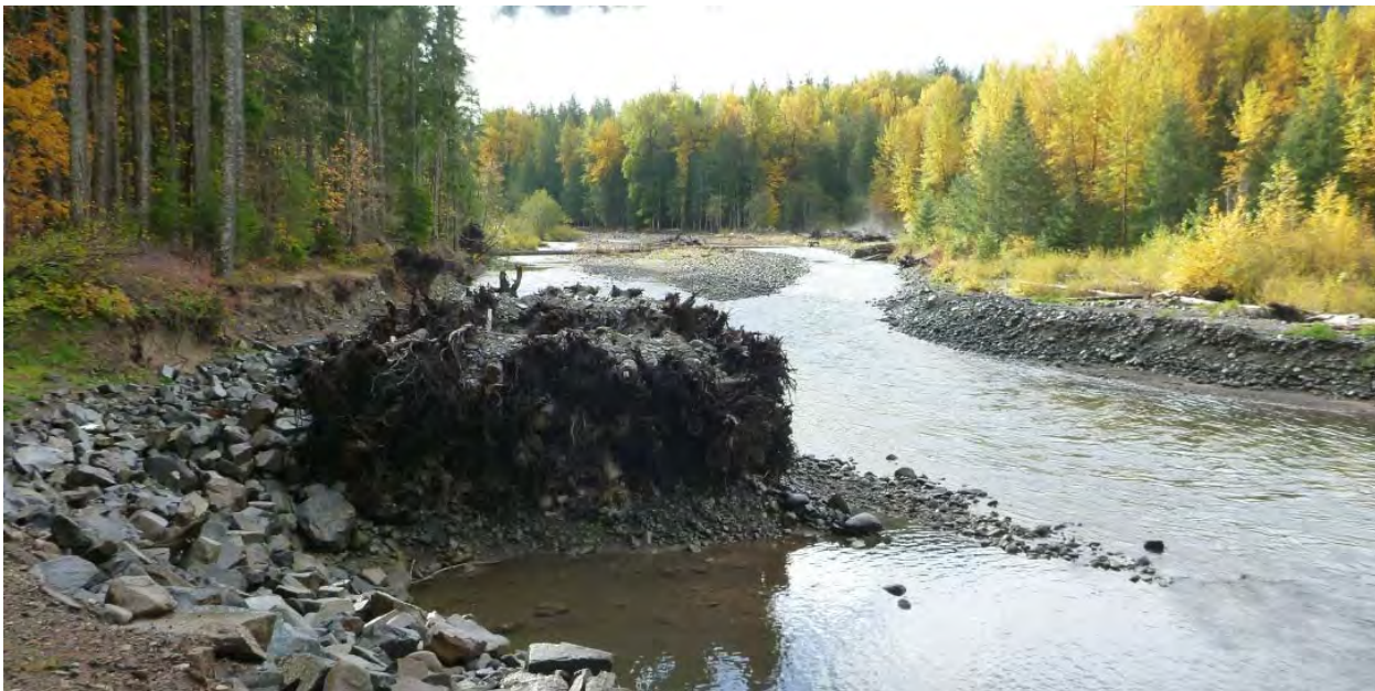
Figure 10. Large engineered log jam at upstream of FS Road 23 repair near RM 21.
