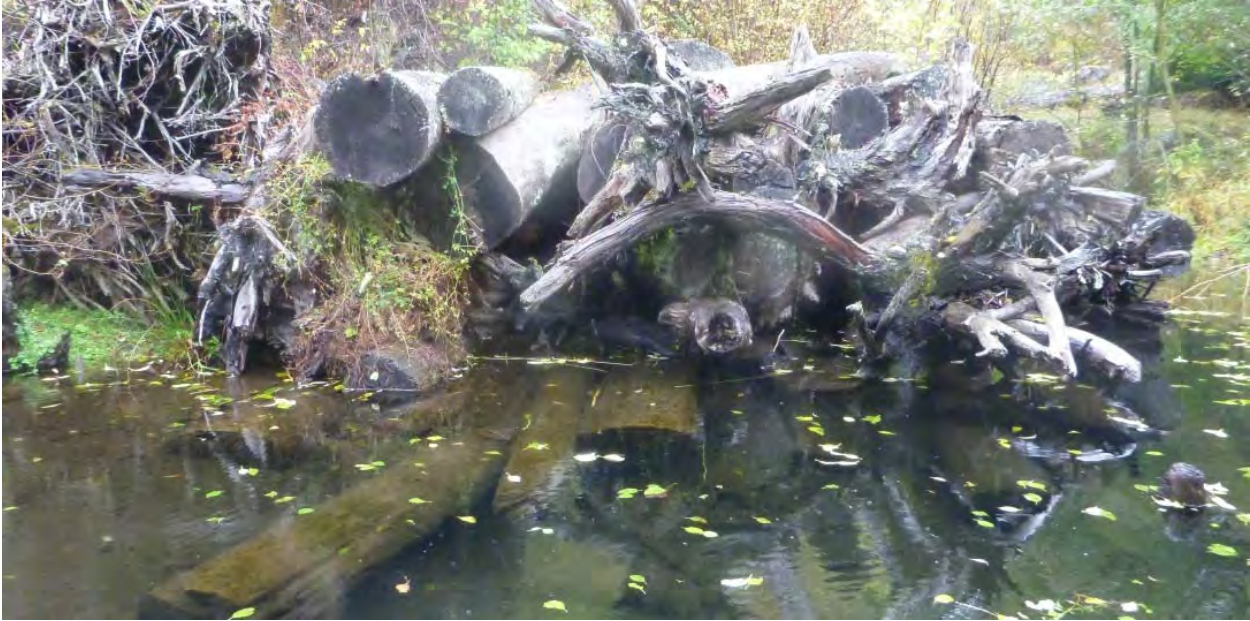
Figure 11. Older engineered log jam placed along FS Road 23 near RM 19 (now in abandoned oxbow).
