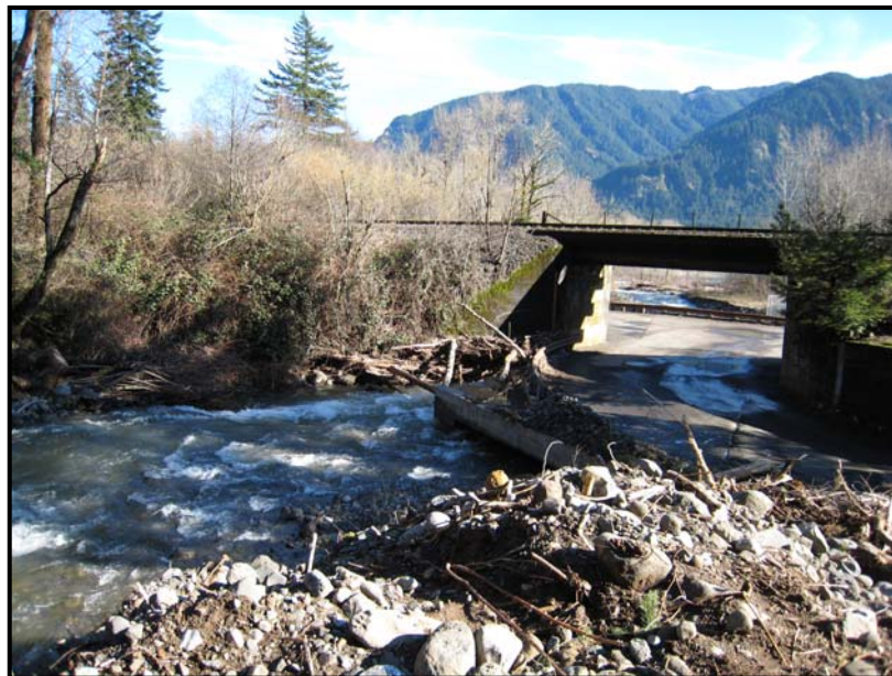
Figure 9. Railroad Culvert and Roadway after 2006 High Flows (January 2007).
