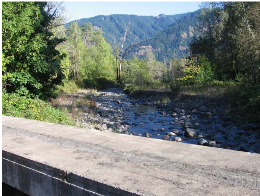
Photo 24 – Looking downstream from Beacon Rock Moorage Road culvert into the seventh reach, bed is primarily coarse cobble with some small boulders
