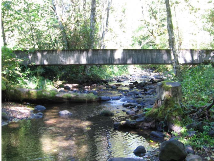
Photo 5 – Deflector log structure right bank and cabled rootwad on left bank immediately below Woodward Creek Road bridge
