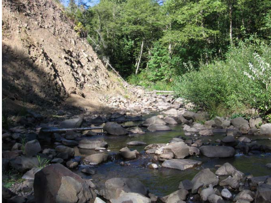
Figure 12 Eroding Bank Near Downstream End of Reach 4
