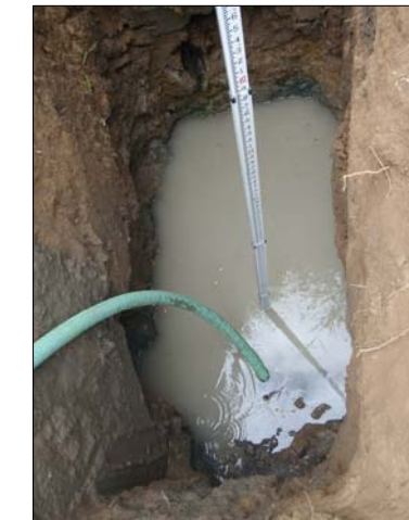
Groundwater Pump Test - Depth Varies 4' to 10' After Testing a 4" PVC Standpipe Will be Placed and the Hole Backfilled
